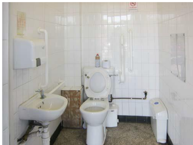
Disabled toilet showing missing tiles
