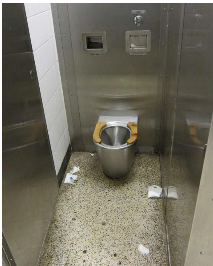
Female toilet showing damaged seat
